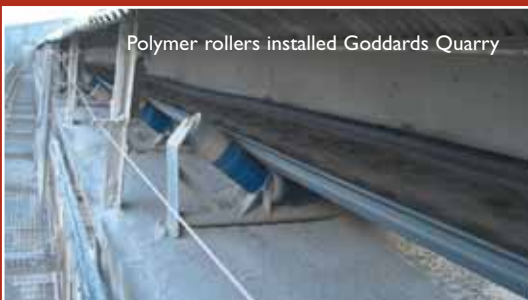
Polymer rollers at Brett Aggregates
