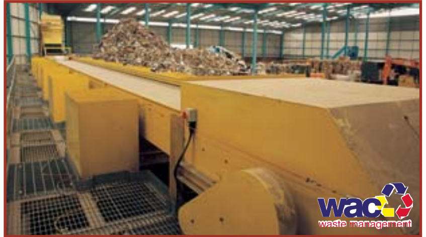
▲ Waste Sorting System supplied to WAC Waste Management
