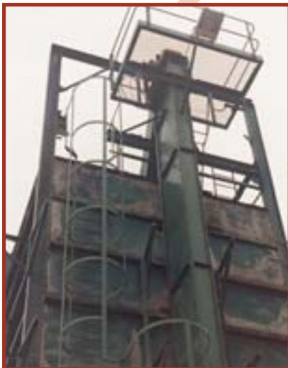
▲ Complete bucket elevator installation
