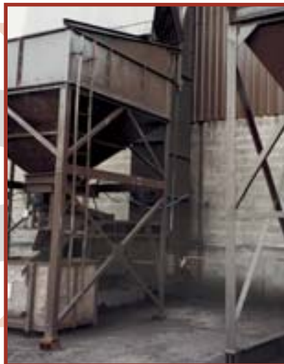
▲ Hopper feeder and elevator system supplied to G Owen & Sons Ltd.
