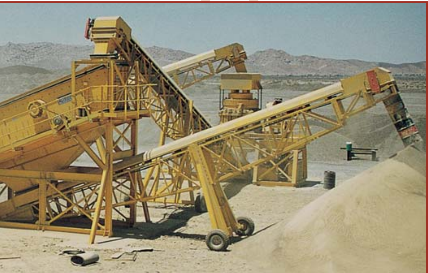
▲ Conveyor incorporated in Crushing and Screening Plant Operation in Middle East
