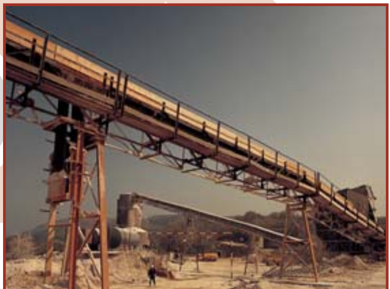
▼ Replacement gantry with gravity take-up unit
